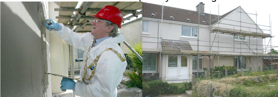
St. Ives Town Mayor helps with overcladding in the home health project at Carnstabba
