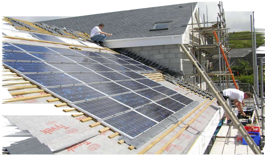
Fitting of solar panels on the roof of Pendeen Parish Member's Institute
